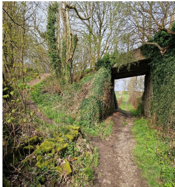
Photo 6: Application route turns sharply east-south-easterly and leads under the disused railway line, which is now a permissive bridleway called the 'Meltham Greenway'. A worn path leads up the embankment and links the Application route with the permissive bridleway. The surface is waterlogged in parts and predominantly made up of earth and stone (Photo direction is west-north-westerly)
