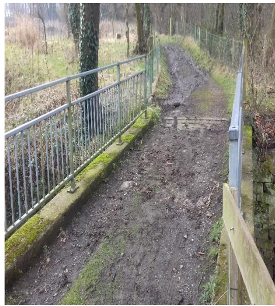
Photo 8: Application route leads over Meltham Dike watercourse via a brick bridge with railings on either side.
